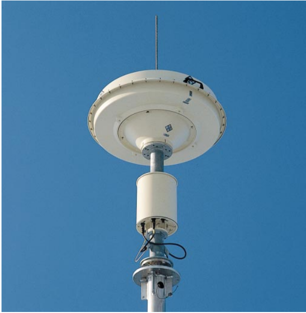
FIG 4 Antennas ADD190 (top) and ADD071 on common mast Photo 42 477/1
